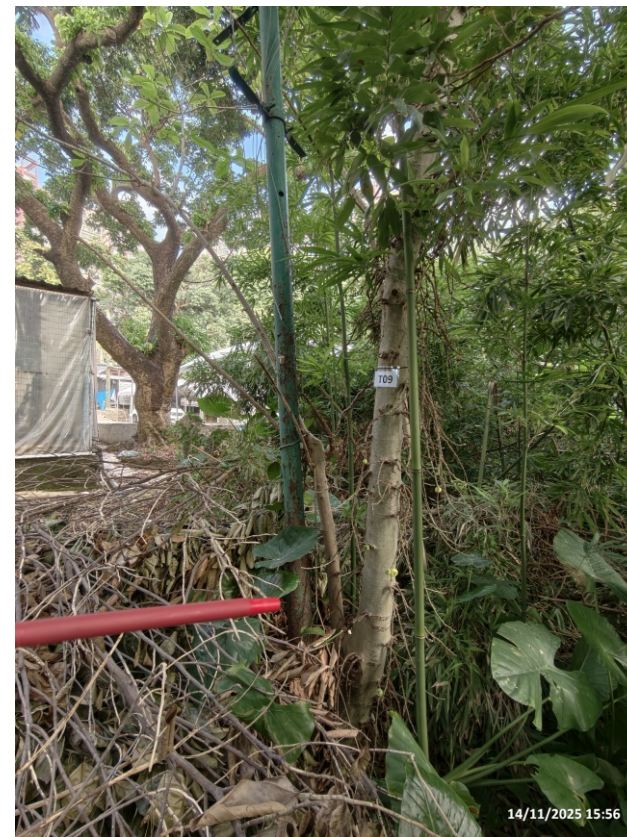
T09 (F) - Trunk Conflicted with Telephone Pole
